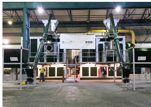
The standard dual retort plant has a footprint of just 6000sq ft for the production of up to 20MWe.
